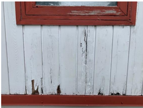
Craig-Klawock Rotting Siding
