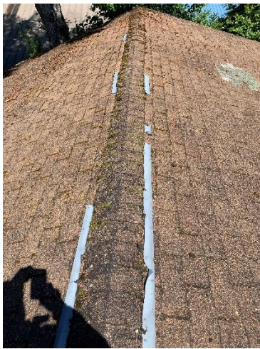
Craig-Klawock Roof of youth center—needs to be replaced
