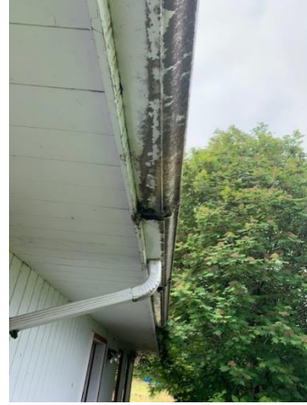
Craig-Klawock Gutters on church overrunning because they're plugged
