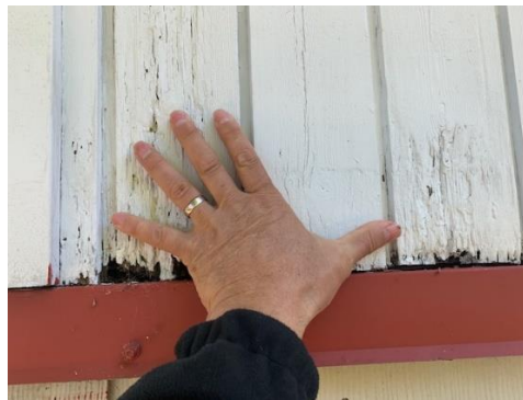
Craig-Klawock Rotting siding
